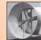
Battery Room Exhaust Fan (User Supplied)
